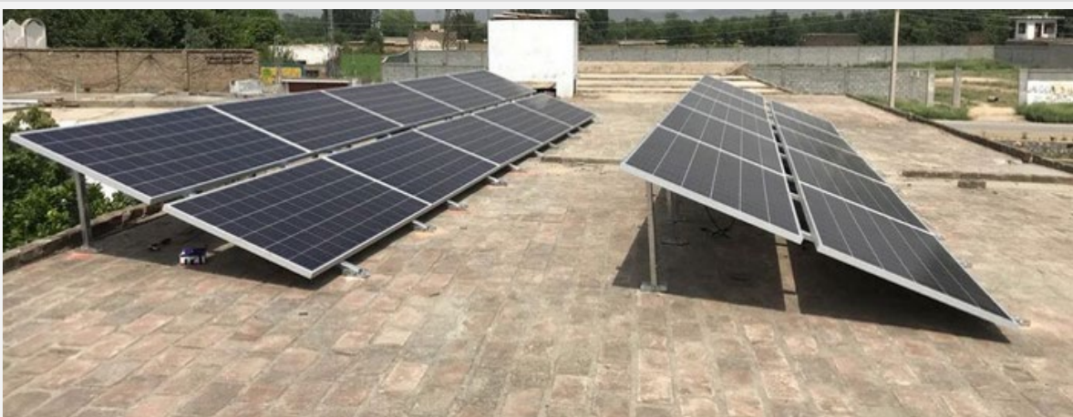
Solar installation at remote location (Sakhakot) in Northern Pakistan.
